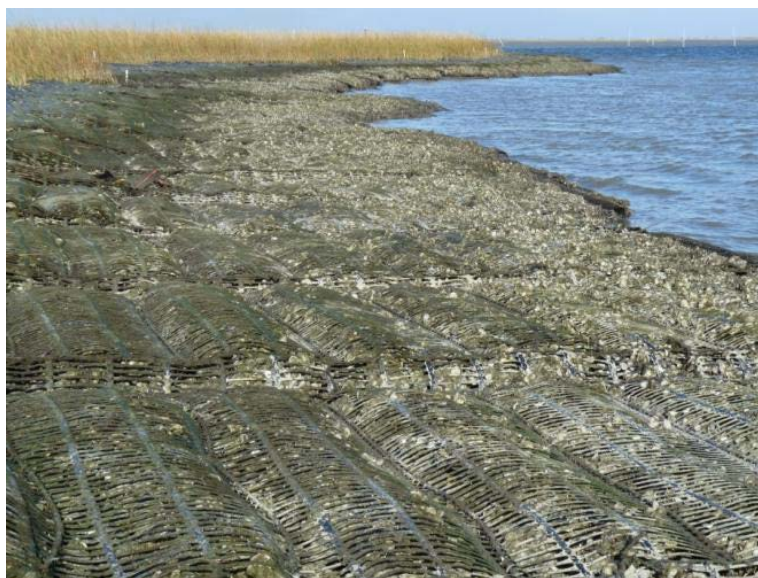
Figure 3. Gabion mats with oyster shell used to restore fringing oyster reefs on the north shore of Terrebonne Bay, Louisiana.
